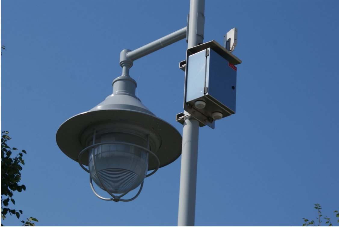
Closeup of 33W LED Light fixture with ballast
