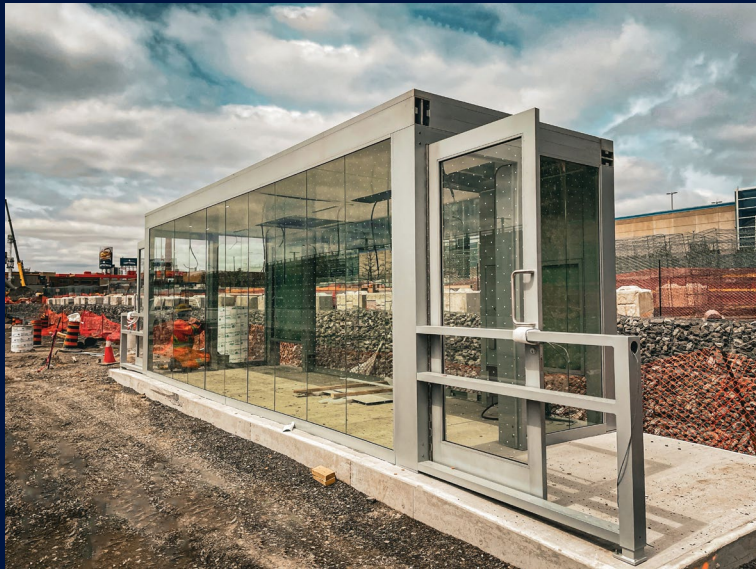
New platform shelters on the temporary platforms will serve passengers during construction
